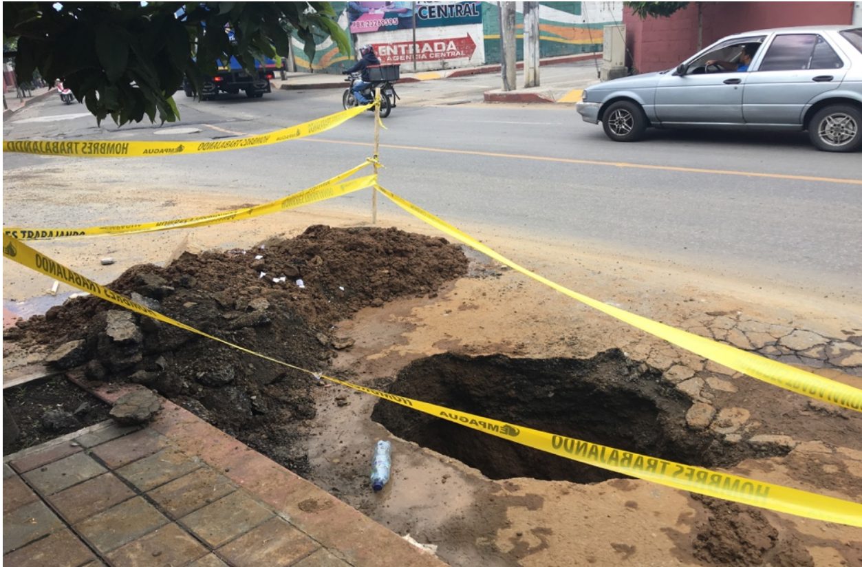
Yellow tape cordons off July 2015 sinkhole in Zone 6, a few blocks from the AHPN. Author's photo.
